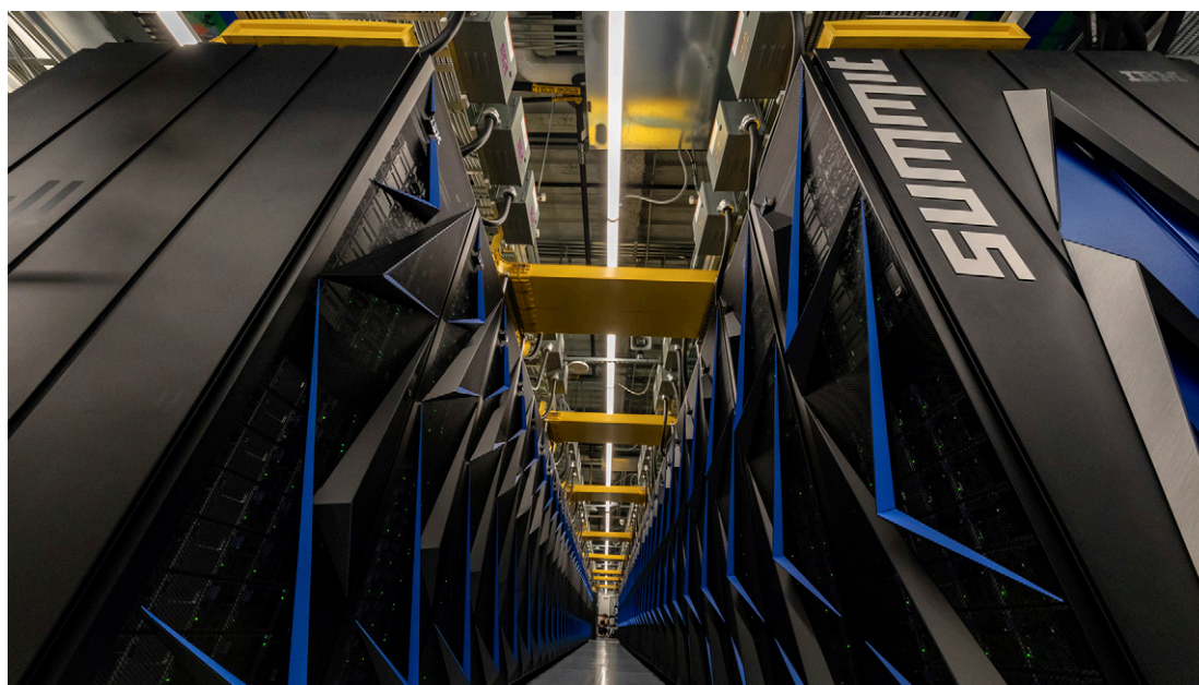
Rows of cabinets hold incredible processing power for one of the world's best supercomputers, Summit, at Oak Ridge National Laboratory in TN. Exascale computing will surpass these existing computers by leaps and bounds. Image credit: Flickr/Oak Ridge National Laboratory, licensed under CC BY 2.0 .
